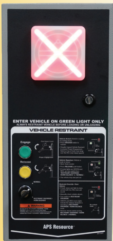
PLC-based control panel with red/green composite light
